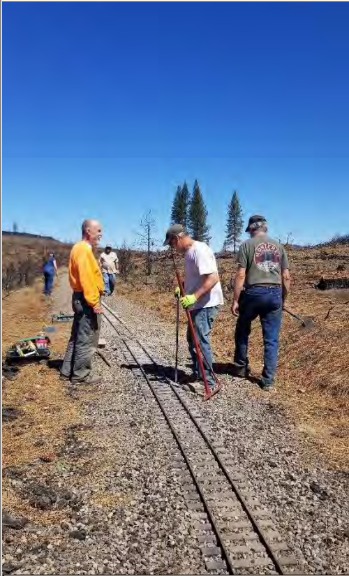
North end fire cleanup
